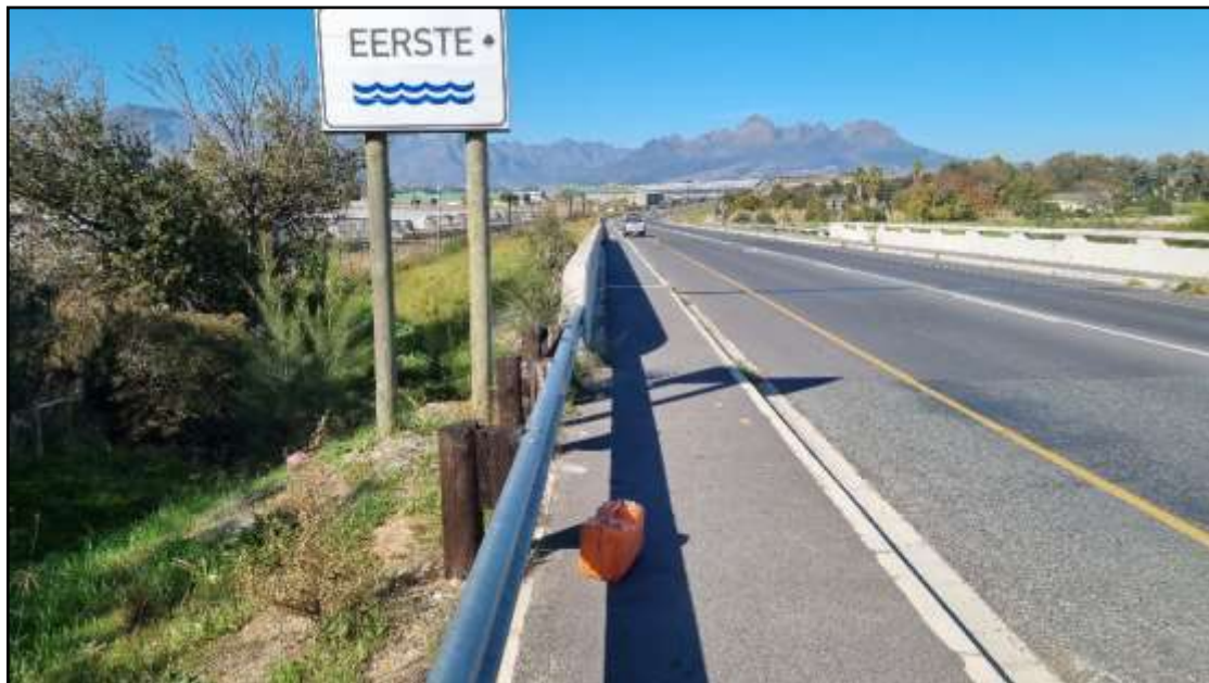
Photo 1: The road surface of the Annandale Road Bridge, viewing from north to south
