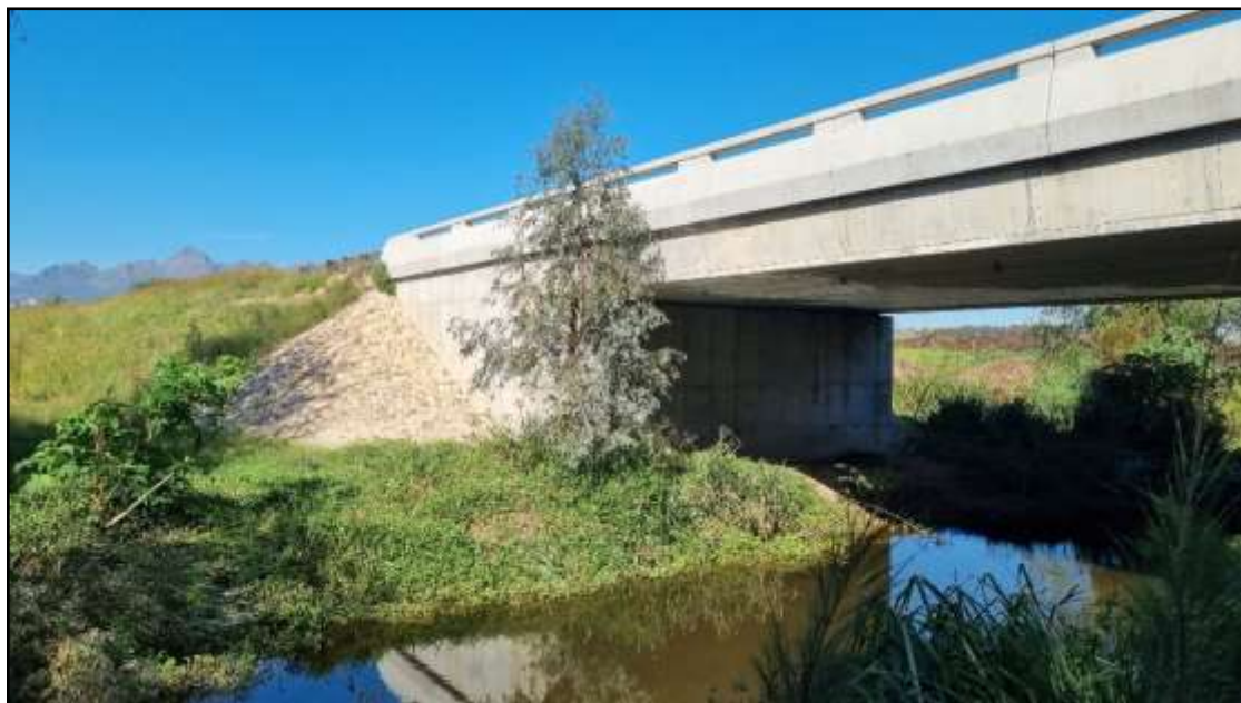
Photo 3: The left-hand abutment of the Annandale Rd Bridge, viewing from the intake side of the bridge. (Note: Left and right banks of rivers are always referred to as viewing from up- to downstream)
