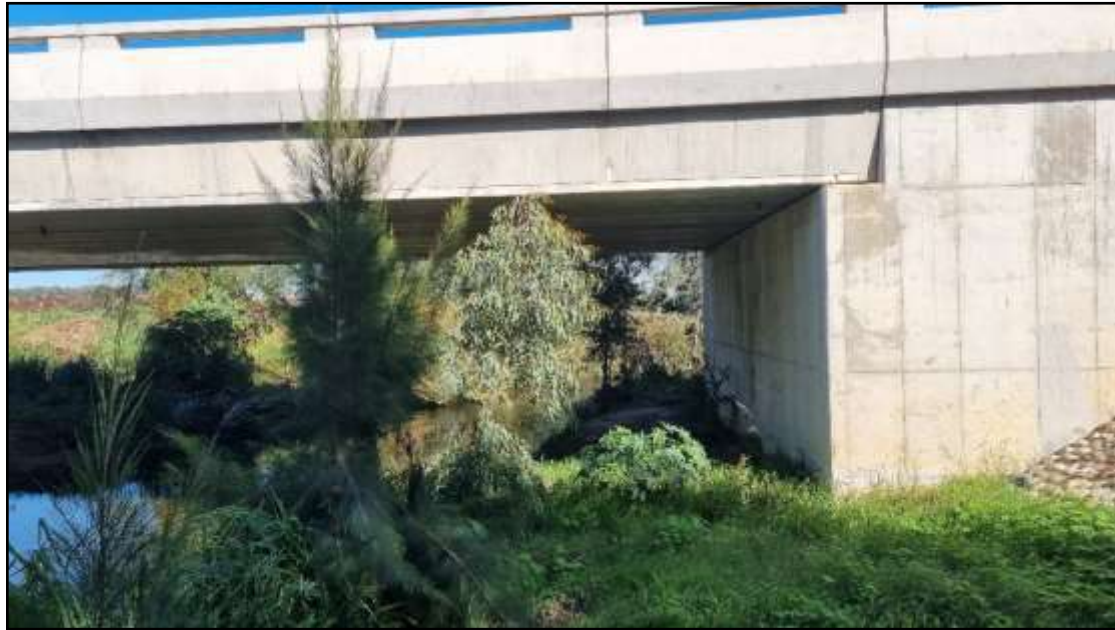
Photo 2: The right-hand abutment of the Annandale Rd Bridge across the Eerste River, viewing the intake side of the bridge
